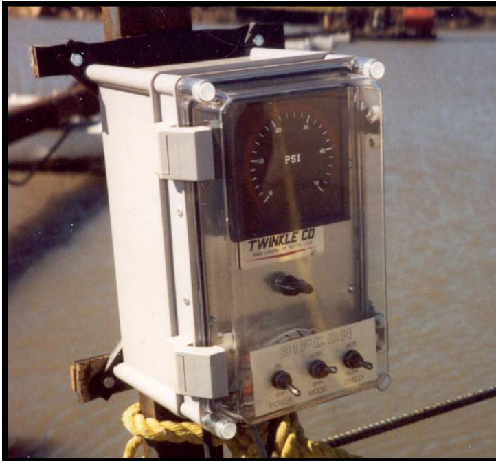
BIPCON control and display enclosure shown in use on a floating booster.
